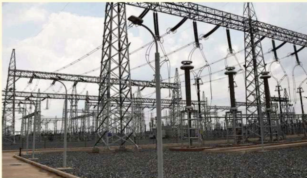
Karuma Hydro transmission lines
