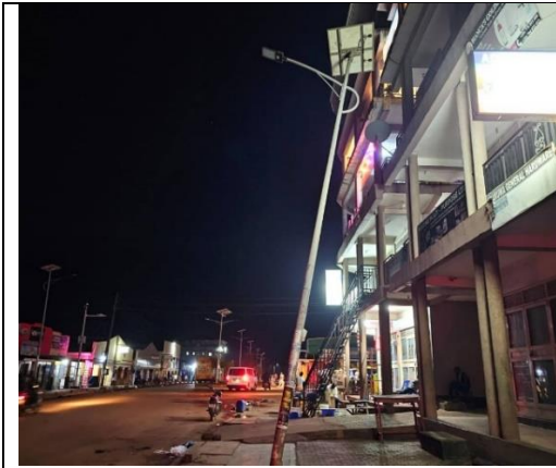
Damaged pole in Lira posing a safety risk to the nearby traffic close to the street pole
