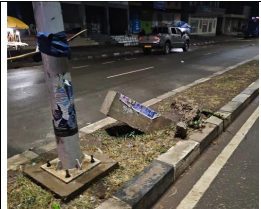
Knocked pole barrier in Mbale; road island width is too narrow – safety risk to motorists
