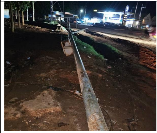
Street pole brought down, and all components stolen at Lira
