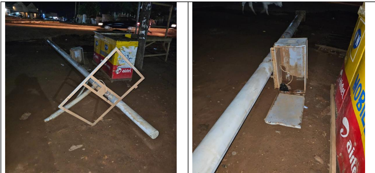
Streetlight vandalised and the solar panels and battery stolen at Lira City at the roundabout of Obote Avenue, Kyoga Road and Soroti Road.
