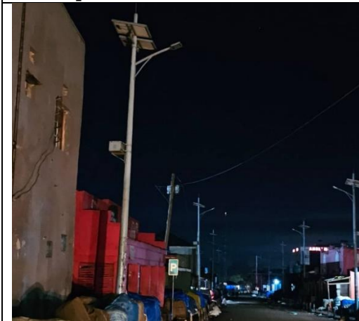
USMID1 Street Lights at Awange Mola Road in Lira were all non-functional
