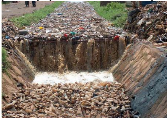
Plate 12: Flooded drainage in Kampala city
