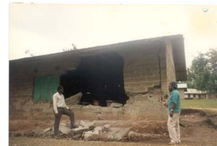
Some walls collapse as a result.
