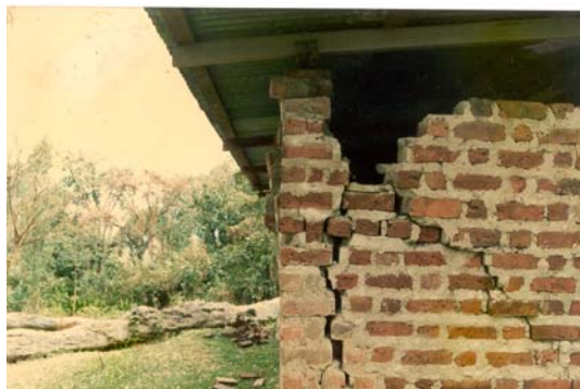
Weak joints especially in corners lead to cracks
