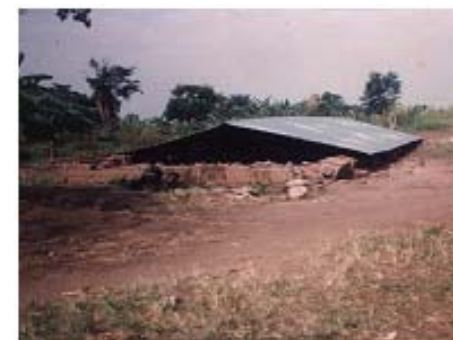
The building may subsequently collapse like the above classroom block in Bundibugyo.
