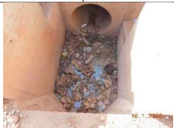
A mix of storm water and solid waste in the channel
